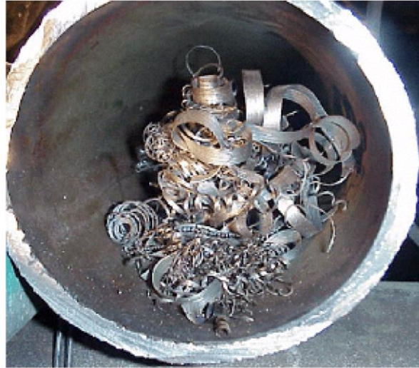
Figure 1. Metal Shavings found in piping following the Fitting Process
